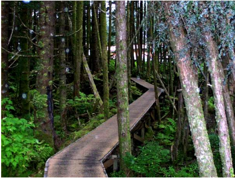
Figure 3 Image of a Port Alexander boardwalk (Alaska Department of Community and Regional Affairs).
